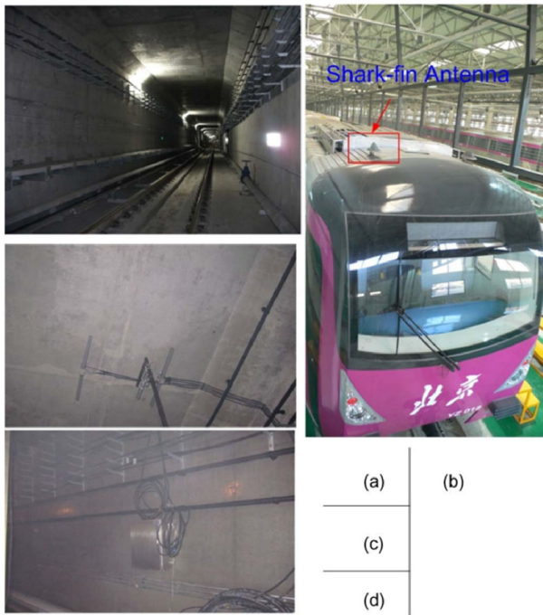
Fig. 10. Experimental setup used to collect data from for the study in [107]. (a) Tunnel where measurements were taken and recorded. (b) Shark-fin antenna located on the measurement vehicle. (c) Yagi antenna. (d) Access point in a section of the tunnel installed on the wall.
