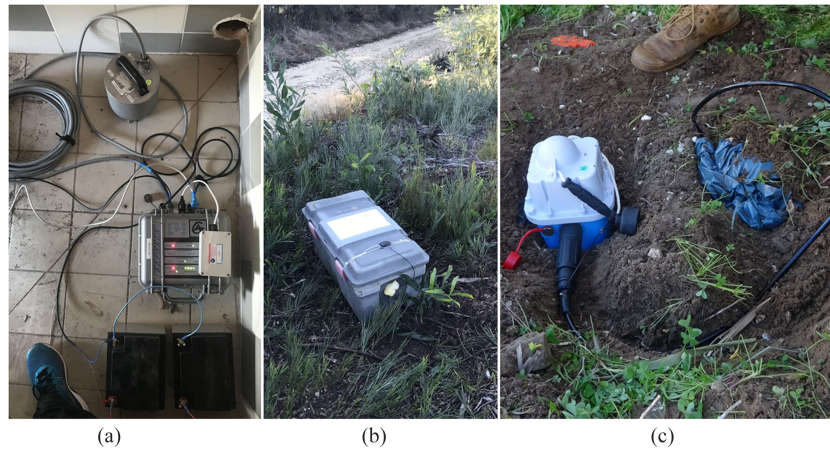
Fig. 6. (a) Broadband sensor and a digitizer installed in a small room at the location labeled PS12 in Fig. 1. (b) and (c) When the instruments were installed outside, the sensors were buried, and all the associated parts (digitizer, disk, and batteries) were placed in a plastic box, as illustrated (b) for the sensor located at PS07 in Fig. 1.
