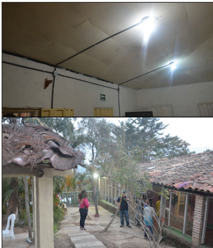
FIGURE 3 – Top: LED Lighting in the Hogar CREA. Bottom: Madres campus and classrooms.
