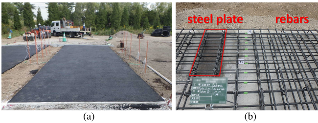
Fig. 7. Pictures of the bridge slab field. (a) Panomeric view. (b) Rebars and the steel plate installed inside the slab.
