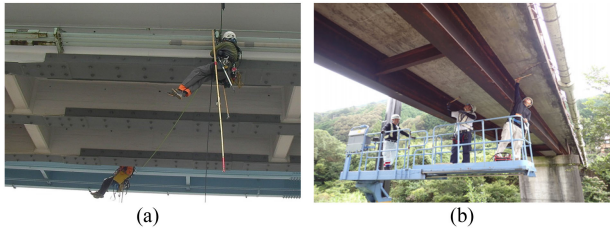
Fig. 1. Example of inspection using (a) rope access and (b) high-location work vehicle for bridge inspection.
