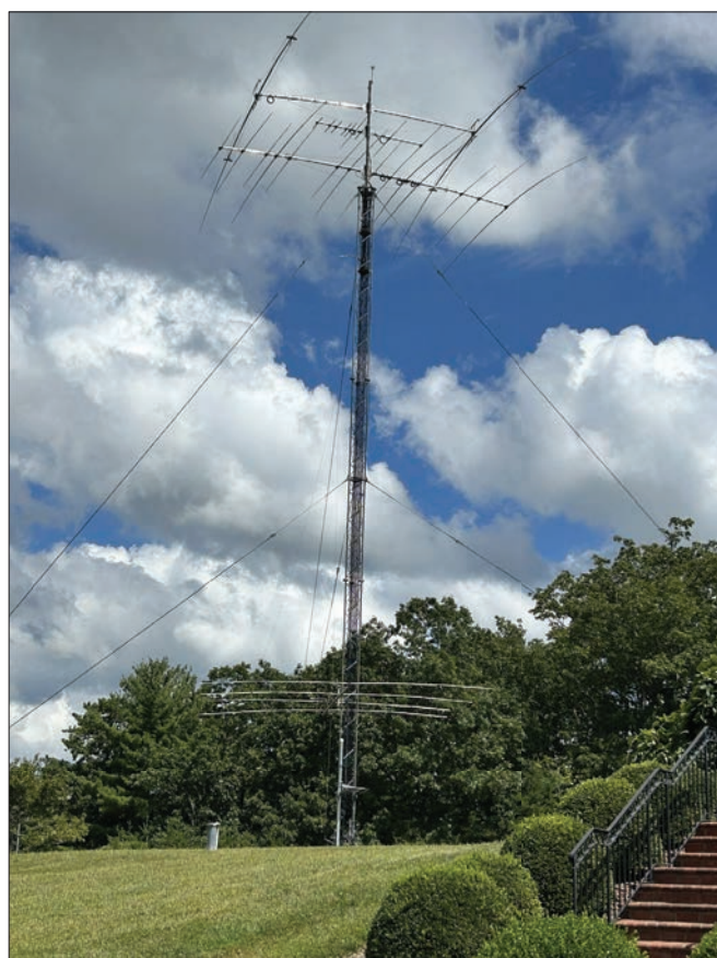
FIGURE 4. Installation of four Yagi antennas on the author's amateur radio tower on a ridge-top at station N9NB in Riner, Virginia. The lowest Yagi is a 4-element tri-band Yagi (10 m, 15 m, and 20 m bands) fixed towards Europe (NE direction), and the largest Yagi (by number of elements) is a rotatable tri-band Yagi at a height of 65' (shown here beaming towards Asia in the NW direction). The smallest Yagi is a dual-band VHF/UHF (6 m and 2 m bands) at a height of 68' that is also rotatable on the same mast, and the tallest Yagi is a rotatable two element mono-band 40 m Yagi at a height of 70', also rotated on the same mast. The height of a Yagi above ground and the nearby ground slope both impact the elevation angles with the greatest antenna gain. (Photo (c) T. S. Rappaport).
