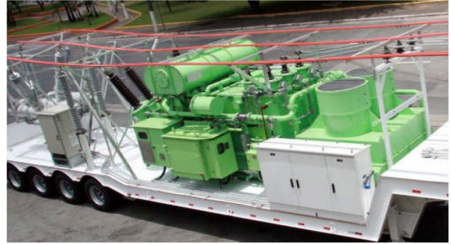
Fig. 7. 138-kV compact mobile substation filled with a high oleic sunflower-based dielectric insulating fluid.
