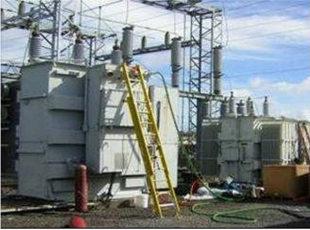
Fig. 8. 69-kV transformer being prepared for retrofilling in the field with a high oleic sunflower-based dielectric insulating fluid.
