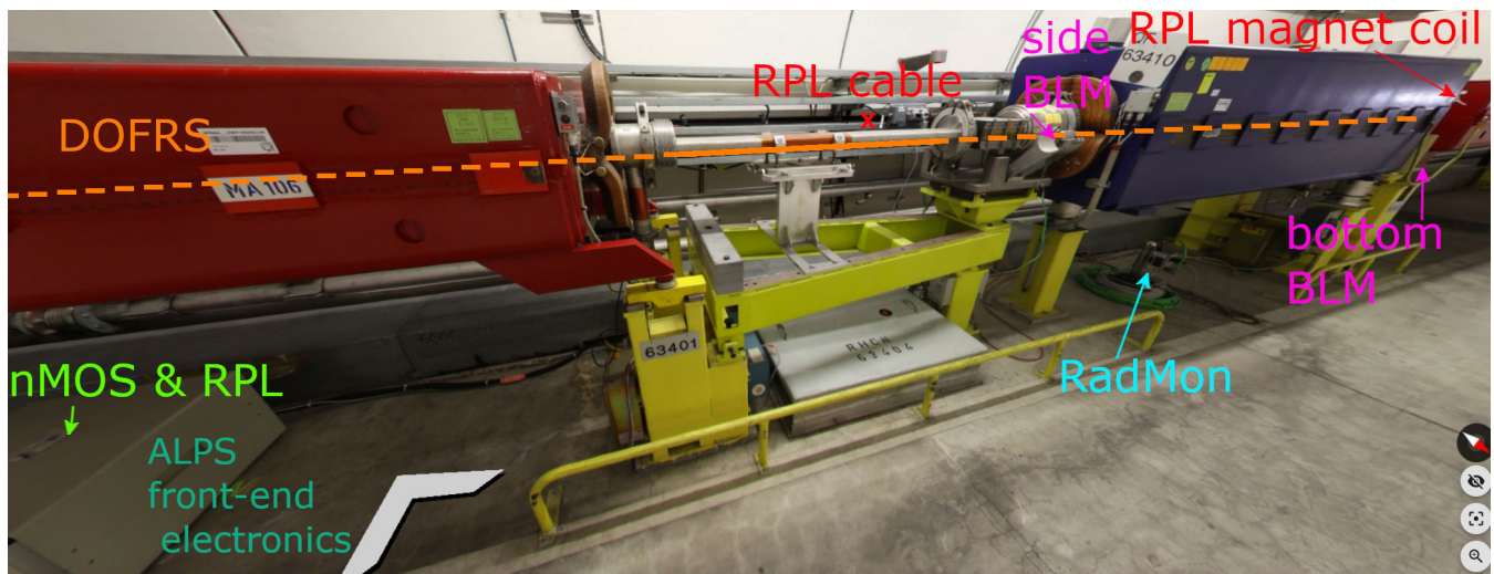
Fig. 4. Standard positions of the radiation sensors in the SPS arc sections, with the electronic rack of the ALPS system (with nMOS dosimeter on top, \sim 0.9 -m distance from the beamline), directly exposed to the mixed-field radiation. Behind the magnets, at the cable tray ( \sim 1.3 -m distance), as of 2021, the DOFRS monitor is installed. Before 2021, the TID was assessed by the RPL dosimeters ( \sim 1 -m distance), in each arc half-period one installed at the cable tray, and one at the magnet coil. Each arc half-period contains one BLM, installed either at the side of the beamline ( \sim 30 -cm distance) or under the first dipole magnet, as in the presented location. In addition, in some half-periods, RadMons are deployed under the magnets.
