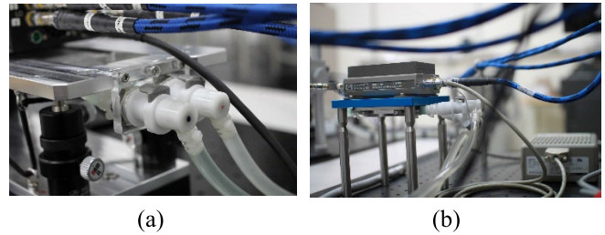
Fig. 6. Cooling system for (a) frequency extenders and (b) common LOs amplifier.
