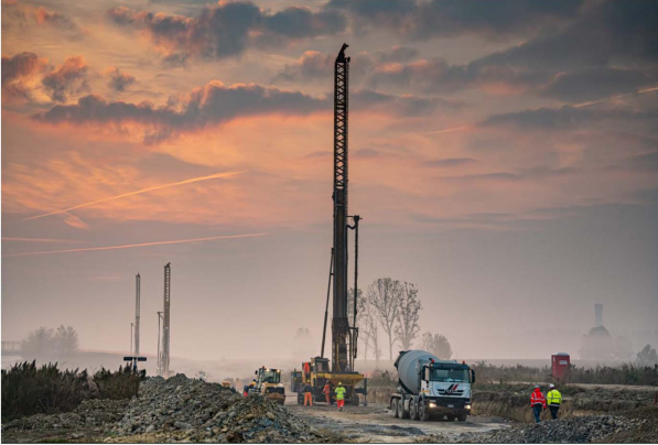
Fig. 2. Here a series of three instrumented rigs can be seen on a building site. This gives an impression of the scale of operations and the relevance of location registered data.
