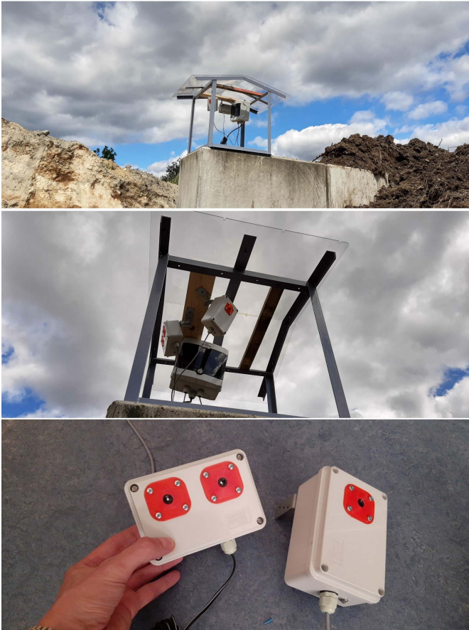
Fig. 9. Real installation of a prototype for measuring landfill surface temperature. The top part shows a view of the whole installation with landfill, the middle part shows a detail of the prototype installation, and the bottom part shows used sensors with adequate IP protection.
