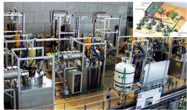
Fig. 9. Image of the TCV's 4.5-MW EC HCD system [87], [88], which is located \sim 30 m from the tokamak center (inside concrete wall). A reference of the plant layout is illustrated in the top right inset.
