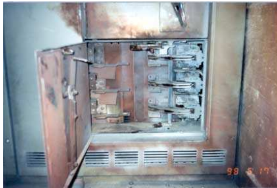
Figure 47—Low-voltage class circuit isolation equipment (front view) where Peter Wiebe was engulfed in the discharge of the arc-flash products (heat, spatter, plasma)
