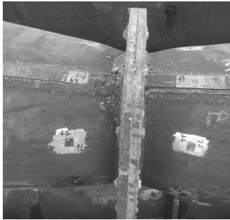
(a) Bulging at the center of the connection
