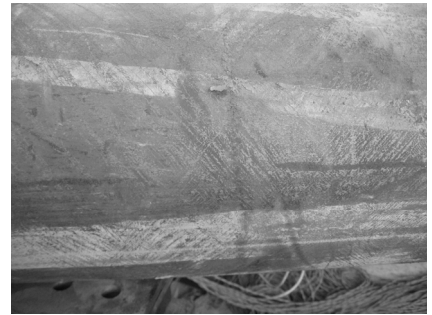
(c) Bulging at the support end
