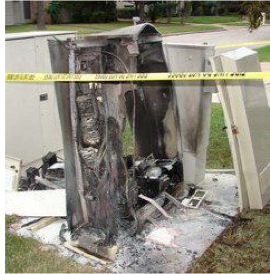
Fig. 8. The result of an Avestor battery fire in an AT&T system.
