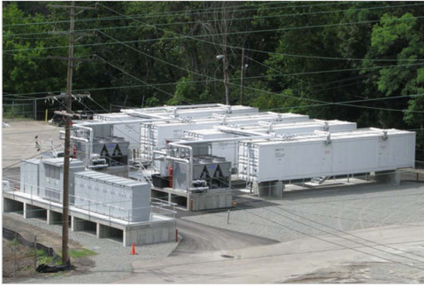
Fig. 12. Energy storage system in Johnson City, NY, uses \text{LiFePO}_4 cells. A similar system has also been installed in West Virginia to smooth the power from the Laurel Mountain wind farm.
