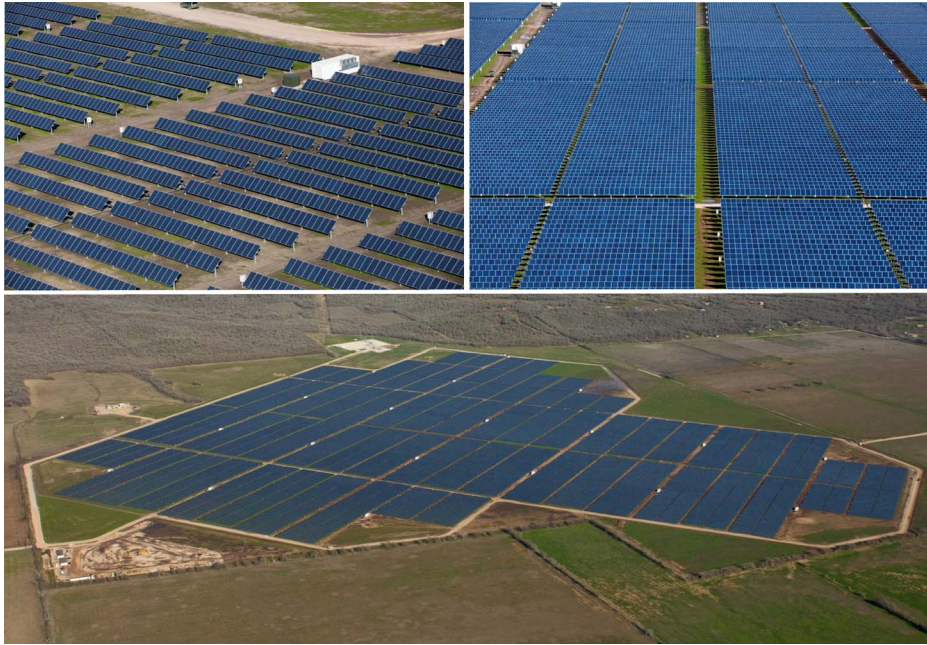
Fig. 13. This Austin Energy solar farm, built by Sun Edison, can generate up to 30 MW, enough electricity to power about 5000 homes. It is located about 20 miles east of Austin in Webberville. Its footprint covers a 380-acre site, and has 127 000 solar panels that track the sun's path. (Photos courtesy of MEMC/Sun Edison.)
